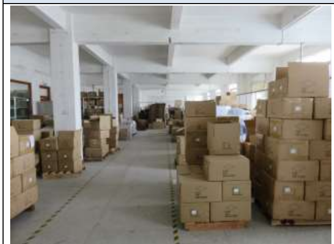
Fire Fighting Equipment
